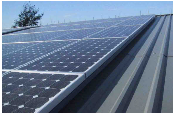
Photovoltaic cells on the roof the WPNSA (c) WPNSA 10
